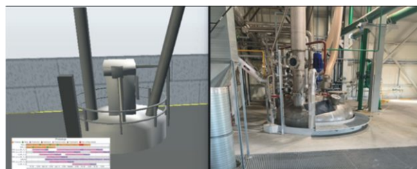
One of the reactors, which is part of a complex of specialized reactors, provides the ability to produce highly specialized resins in both simulation and real-world environments.
